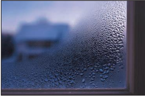
Condensation on the inside of a window-pane.
