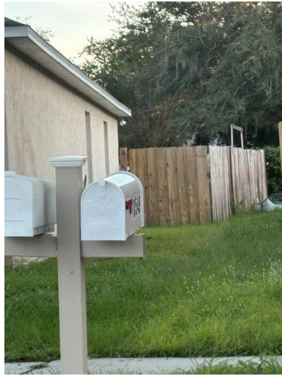
Side fence conditions (slats bowing)
